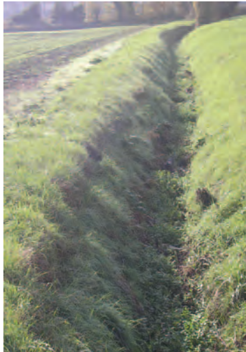
Figure 19.5 Ditch. This is open to the elements and easily choked if not regularly maintained
