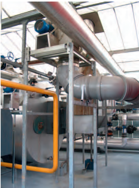
Figure 8.5 CO 2 burner enriches the glasshouse environment, so helping provide an optimum growing environment
